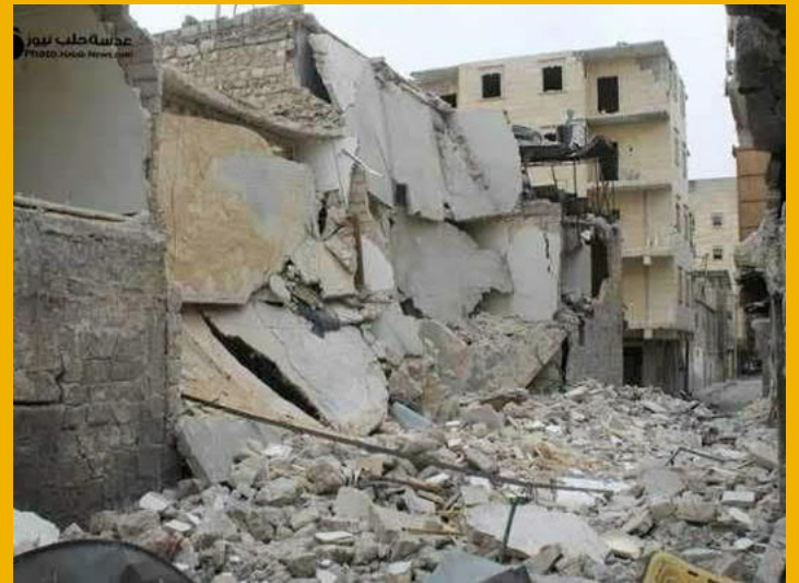
Destroyed house of the Jasser Family in Aleppo city center, 2012, © Adasa Halab News
